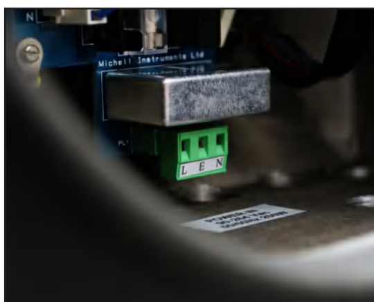
Figure 2 Power Connection Connector
